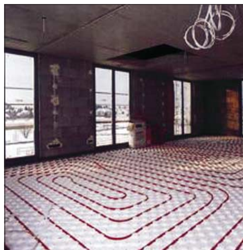
Industrial floor heating
